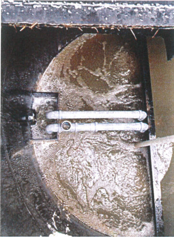
Aeration in Biozone
