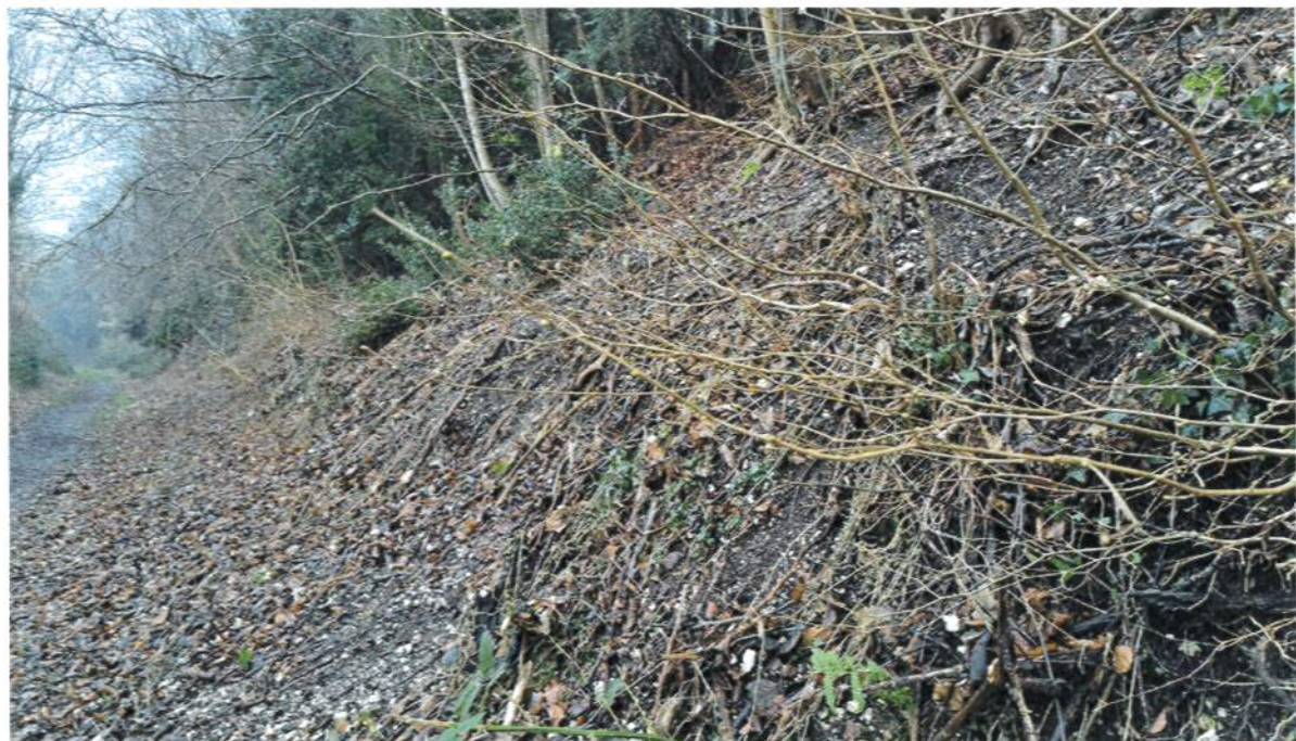
Photo 4 Oversteep topsoil/subsoil accumulation close to base of cutting
