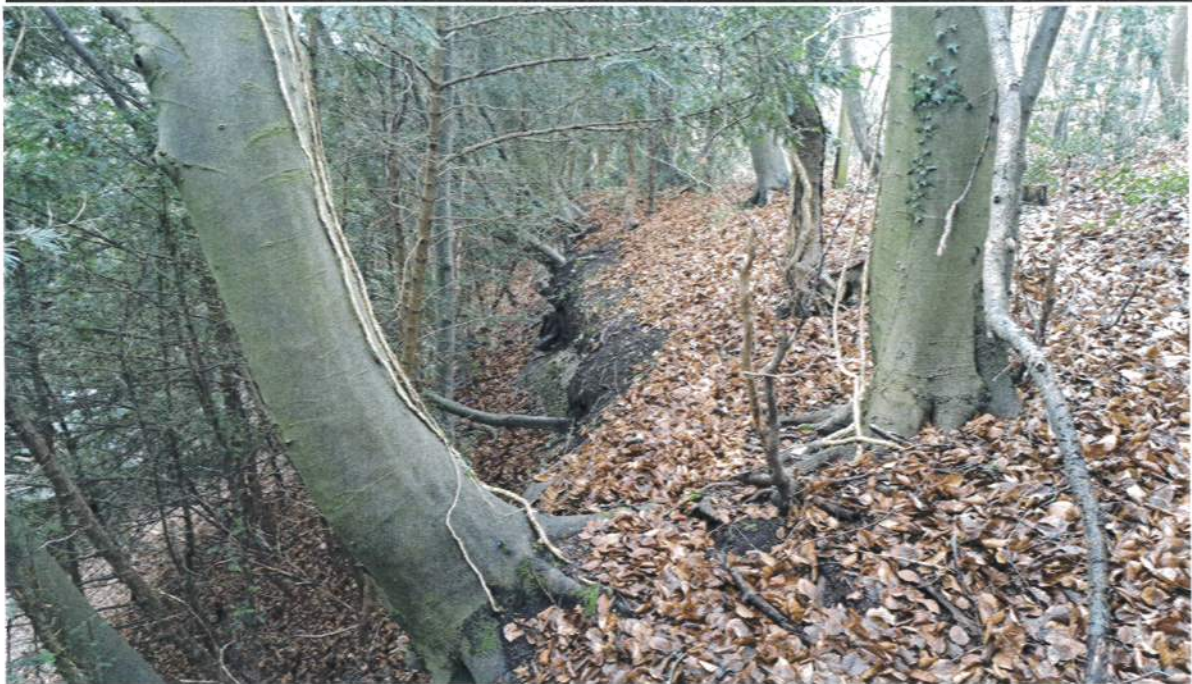
Photo 7 showing tree root systems partially stabilising backscarp at crest of cutting
